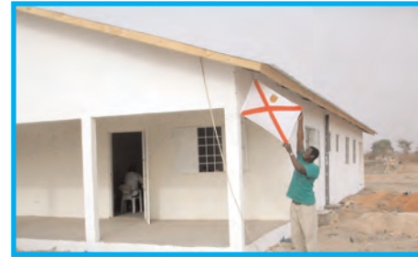
Accommodation Block, completed by local Contractors before the arrival of the Overseas Aid Team. Jersey Flag being put in position!
